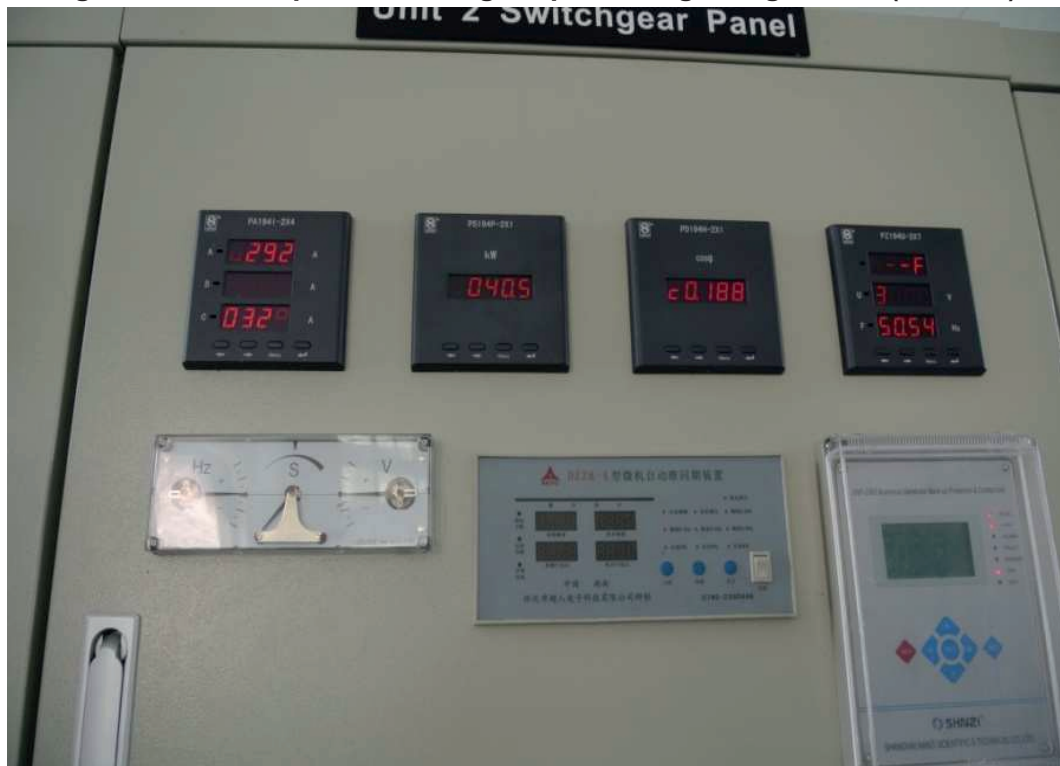
Figure 5: Control panel showing output during inauguration (40.5 kW)
